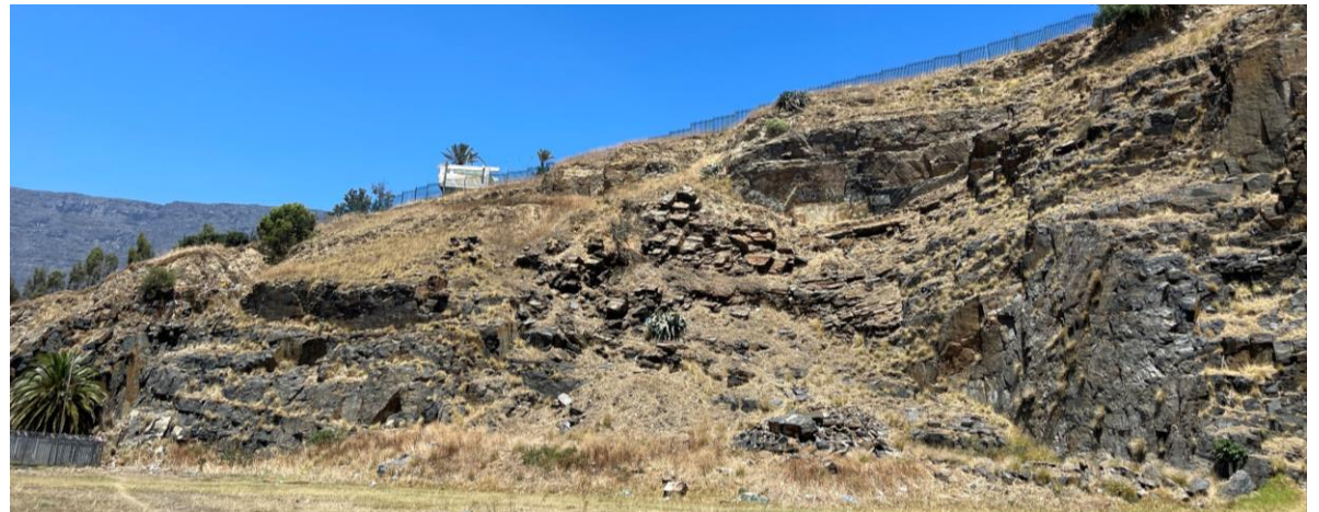
Figure 2.65: Photograph of decayed slope indicating need for intervention (Terra+, 2023).
